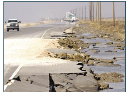
Land Side after Hurricane Ike (2008)
