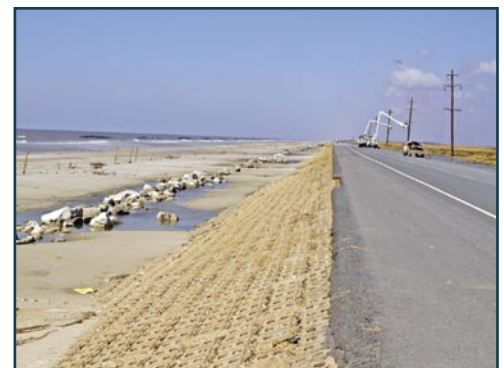
Gulf Side after Hurricane Ike (2008)
