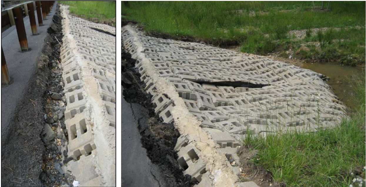
Figure 18. Photographs of ACB Installation at Grover's Mill Dam Showing Armoring Units Damaged from Inadequate Transition Details at the Top of the Installation
