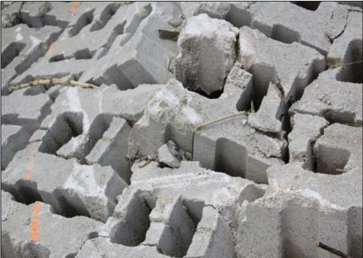
Figure 10. ACB Armoring on Portugués Cofferdam Damaged from Debris Impact (Concrete Jersey Barriers and Concrete Slabs).
