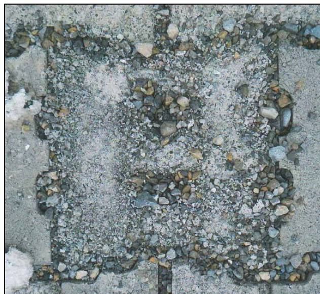
Figure 12. Photographs of Deteriorated ACB Blocks Due to Poor Quality Control during Manufacturing
