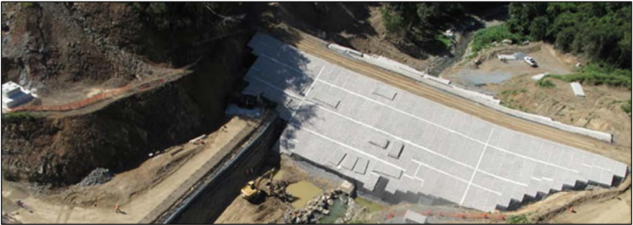
Figure 3. Photos Showing Installation of ACBs on Portugués Cofferdam, Puerto Rico (Photos Courtesy of Jacksonville District USACE)
