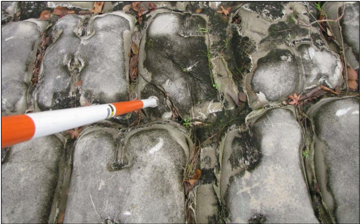
Figure 15. Photographs Taken in 2015 Following a Overtopping of Forest Lake Dam during Hurricane Joaquin Showing Condition of Fabriform ACB System Installed in the 1980s
